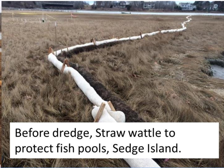
Before dredge prep, coir fiber roll to protect pool & SET, South Middlebridge.
